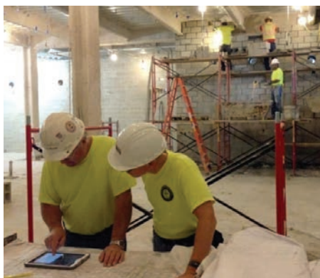
Figure 1. Bricklayers constructed the masonry on this new laboratory building using BIM technology and tablet computers.
