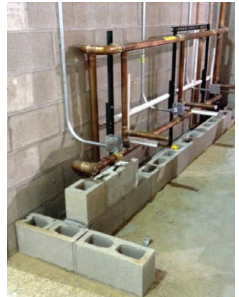
Figure 9. The BIM model made it possible to prefabricate the toilet room plumbing assemblies on steel strut racks to conserve space on the jobsite. The plumbing racks were integrated into the block walls per the coordination model.
