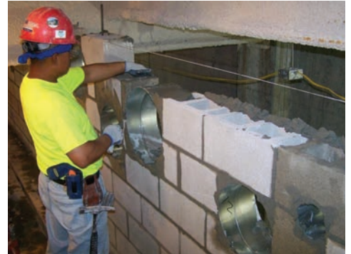
Figure 6. A bricklayer installs mechanical duct sleeves at precise locations per the BIM model, as he constructs the masonry.
