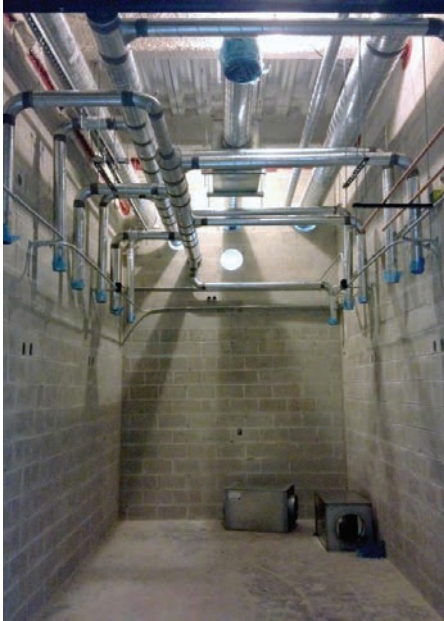
Figure 10. Upon completion of the masonry work, the MEP trades were able to easily install their pipes and ducts without cutting through the masonry due to the well-coordinated sleeve penetrations.
