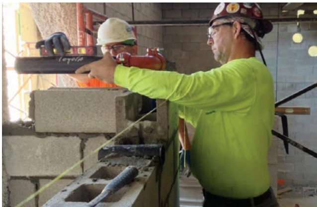
Figure 8. A bricklayer (left) works in alongside a pipefitter (right) to simultaneously construct the block wall and the plumbing contained within it.
