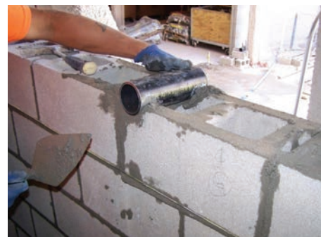
Figure 2. The bricklayers worked alongside the MEP trades to install pipe sleeves through the masonry walls as they were constructed, per the BIM model.
