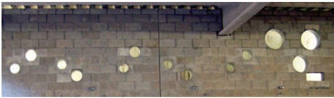
Figure 7. As the concrete masonry was constructed, the bricklayers installed 468 sleeves for HVAC, 69 sleeves for electrical, 159 sleeves for mechanical pipe, 257 sleeves for fire protection, 231 sleeves for plumbing, 343 sleeves for water, and 10 sleeves for miscellaneous, resulting in a total of 1,537 sleeves in the masonry walls.
